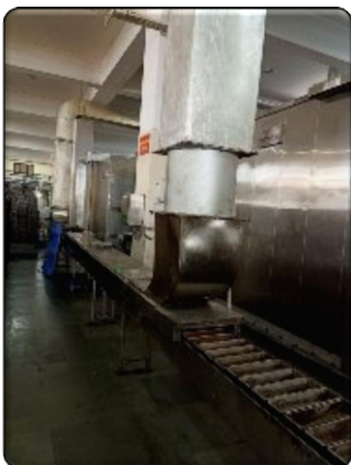
MOULD COOLING SYSTEM
