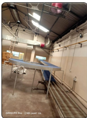
MOULDAR BELD CONVEYOR DRIVES 1 HP
